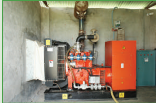
The biogas produced in large commercial biogas plants in poultry and dairy farms is used to generate electricity.
