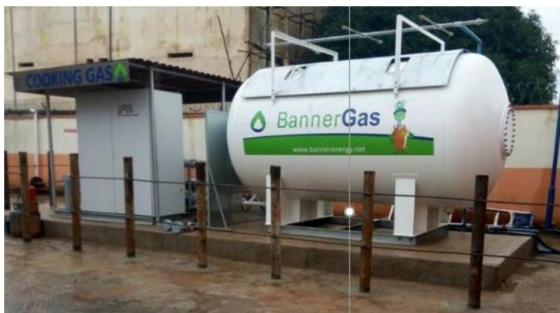
Figure 16: Banner Gas skid (source: Banner Gas)
